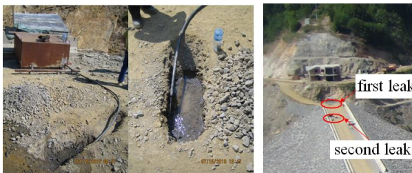
Figure 10. Leakage simulation test with 0.15 l/s
