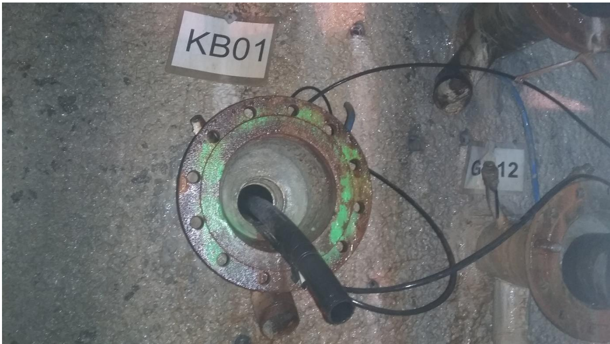
One of the 15 temperature measurement boreholes in the Albula Tunnel II
