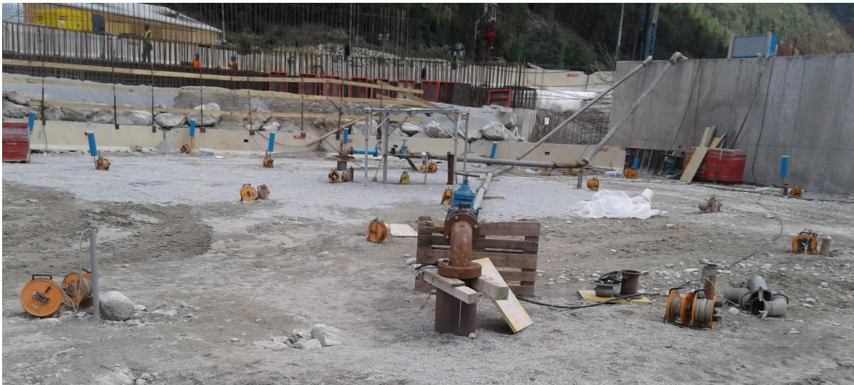
Temperature measuring chains at Brenner Base Tunnel
