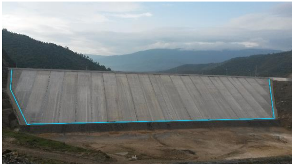
Fibre optic cable along the perimeter of the dam
