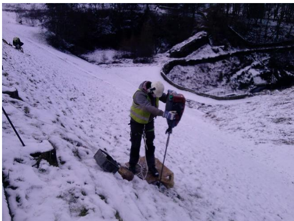
Installation of the temperature sounding at the embankment of the Riding Wood Reservoir
