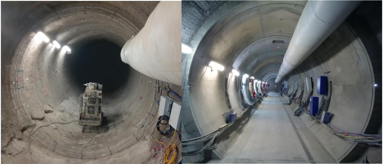
Convergence measurements with optical fibres in the concrete shell of a gallery in the ANDRA field laboratory CHMH(FR)
