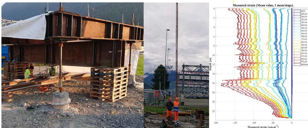
Deformation measurements during load tests of three piles with several fibre optic cables installed in the reinforcement, Bilten (CH)
