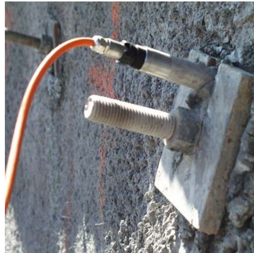
Figure 3.4 Head of the instrumented rod anchor of the nailed wall
