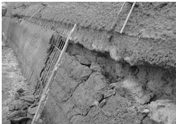
Figure 3. Slumping of the sprayed concrete
