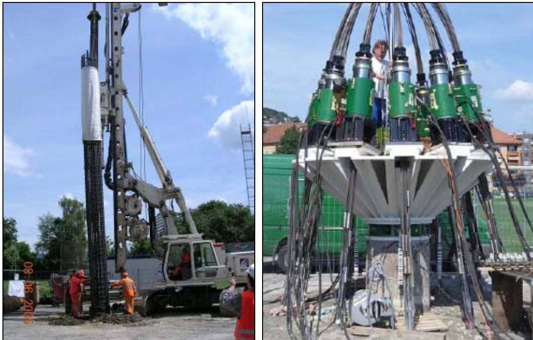
Figure 8: Installation of the pile reinforcement (left) and the top of the pile (right)
