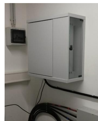
19" AP Sensing DTS device mounted in a flat wall cabinet
