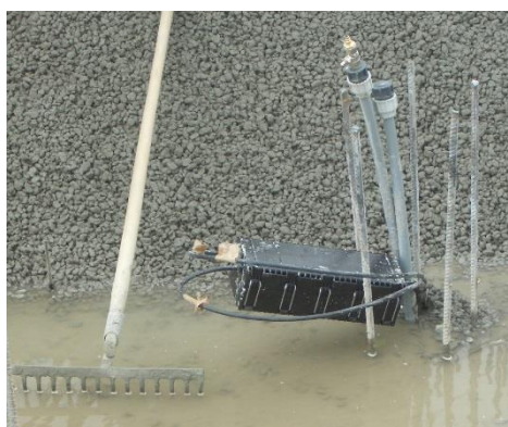
Joint box used to connect cables during installation
