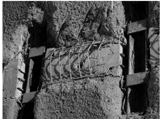
Figure 8. View of the deformable elements installed between the joints of the TH steel ribs.
