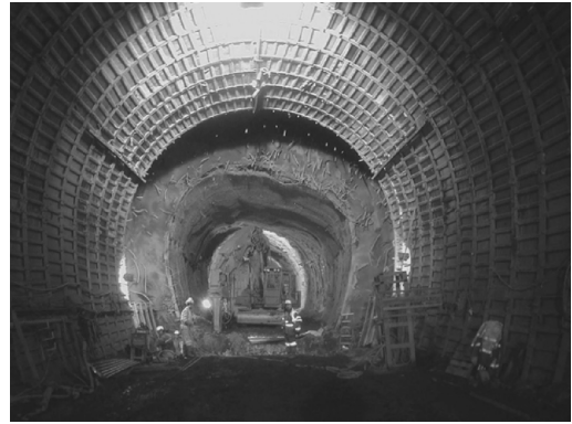
Figure 6. Re-profiling operations of the opening to the original tunnel profile followed by concrete placing behind steel plates.
